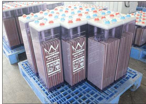
Figure 4-5 A Lithium-ion battery bank similar in size can be expected at typical Metro stations.
