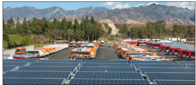
Figure 1-1 Solar Panels at Metro Bus Division 15, Sun Valley, CA.
