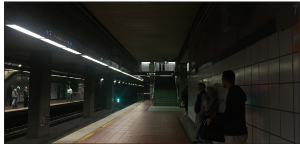
Figure 1-1 Lighting level do not meet MRDC requirements. E (Expo) Line platform, 7th St/Metro Center station.
