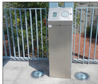
Figure 1-2 Uplighting creates a glare and inhibits passenger visibility. Jefferson/USC station, E (Expo) Line.
