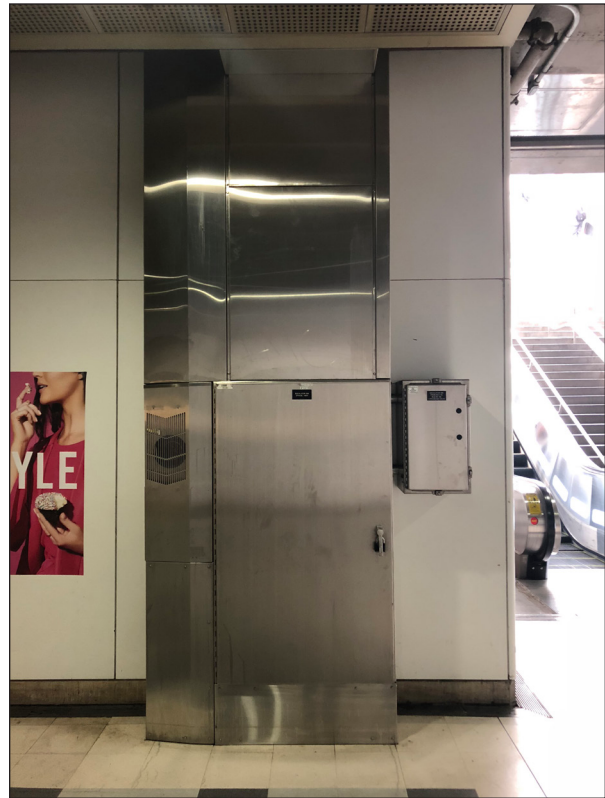
Figure 1-1 Existing retrofitted escalator control cabinet obtrusively located in public space at Pershing Square Station, B (Red) and D (Purple) Lines.
