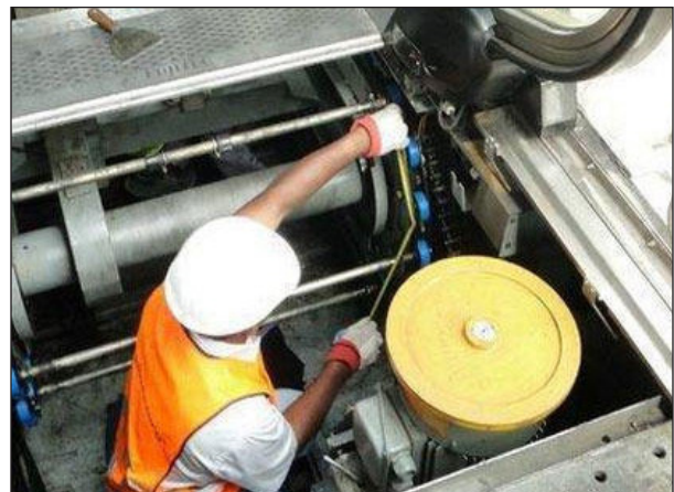
Figure 3-2 Escalator controller located in the escalator machine pit.
