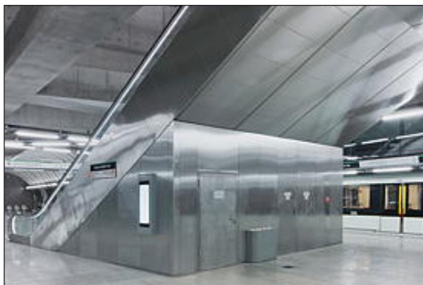
Figure 3-4 Equipment room located in a nearby room, behind and under escalator and stairs. Metro Line M4 station, Budapest Metro.
