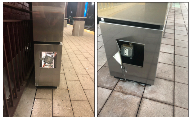
Figure 1-4 Pried open secure electrical outlet
