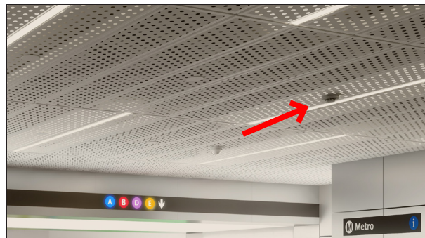
Figure 3-7 Security camera mounted on ceiling with matching finishes.
