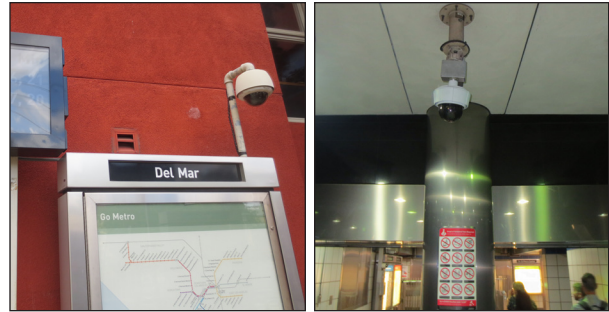
Figure 1-3 Inconsistent mounting of security cameras with exposed conduit.
