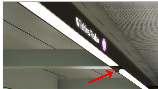
Figure 3-6 Security camera mounted in platform edge lighting signage assembly.
