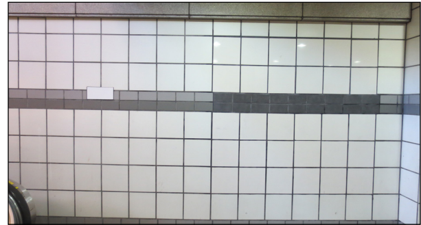
Figure 1-1 Mismatched wall tiles, 7th St/Metro Center station.
