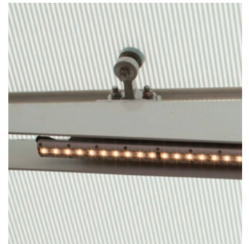
LED Station Lighting
