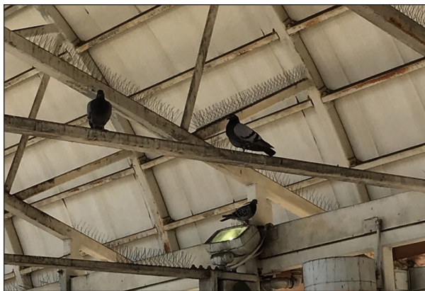
Figure 2-1 Ineffective deterrents at Harbor Freeway Station.
